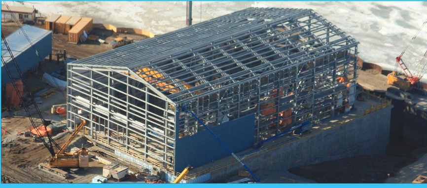
Syncrude Kearn Lake River Water Intake
