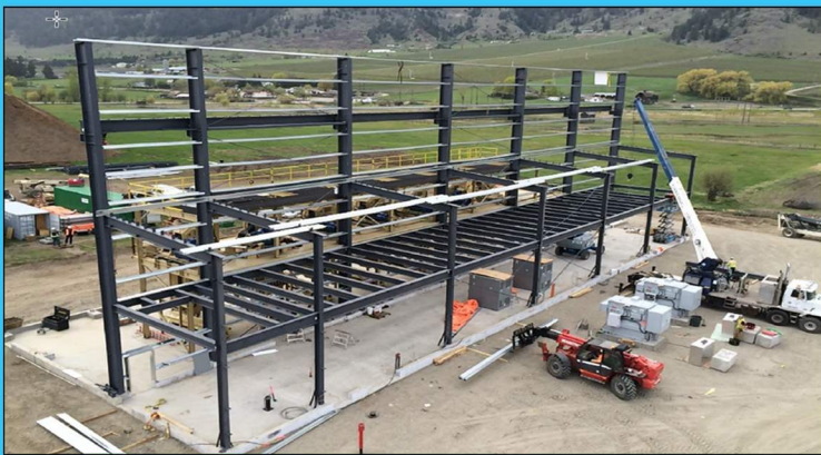
Pinnacle Pellet Lavington Pelletizer & Hammermill Buildings
